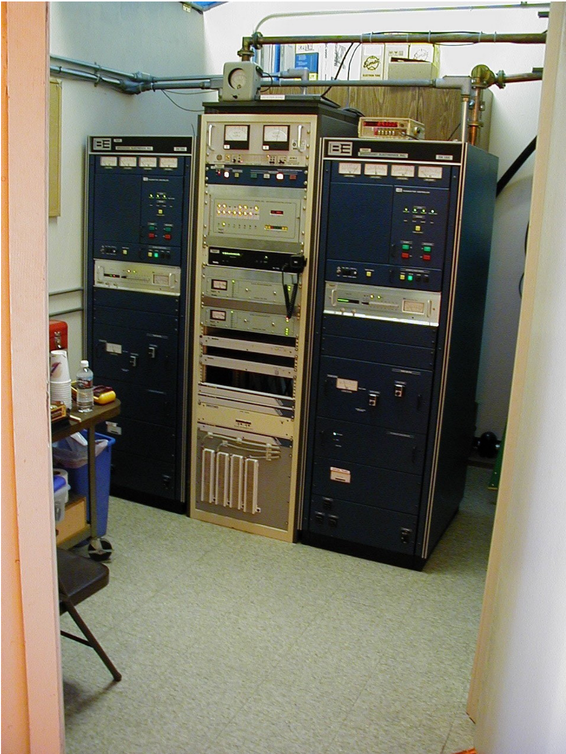
KPCC Transmitter Room
